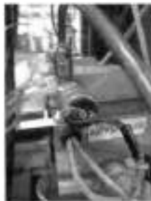
Figure 34 - The air pressure switch
