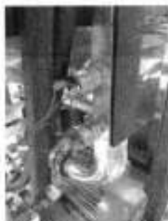
Figure 36 - The air pressure switch
